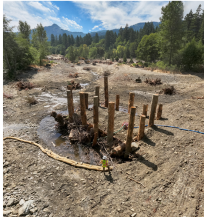
As an example of habitat improvement, the photo shows the installation of a large engineered wood structure at Bull Creek State Park, California. When water flows through the stream the engineered wood jam will help create better habitat by routing water into the floodplain and making a large deep pool for fish to rest in. Photo by Pusher Inc. August 2024.
